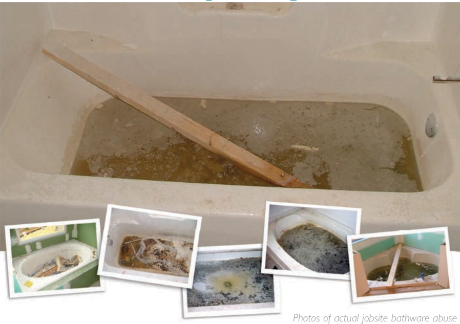
Photos of actual jobsite bathware abuse
